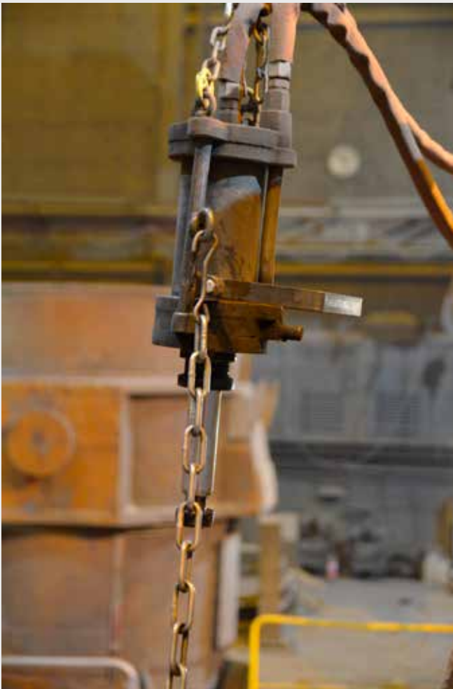
New lifting device for the ladle slide gate cylinder at the rebuilt platform in the steel mill of Smedjebacken.
